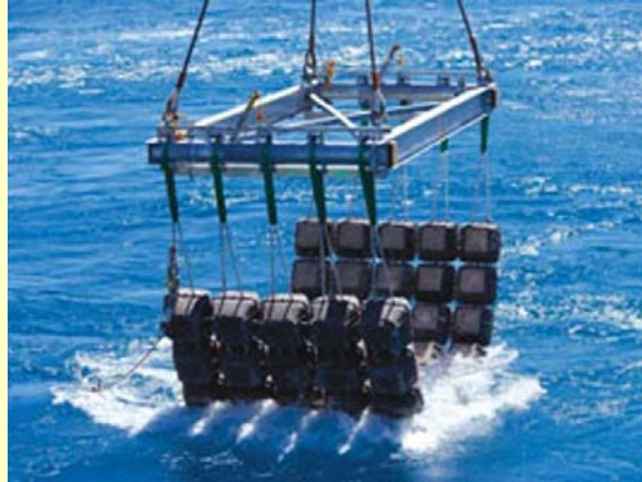
pipeline stabilisation and protection system
